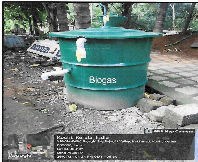
Biogas Plant within the college campus
